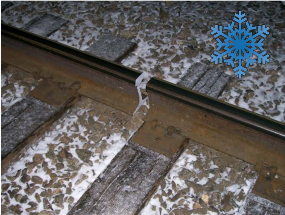
“Pull Apart” broken rail in the winter
